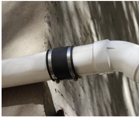
A rubber coupler was used here to connect two pieces of piping.
