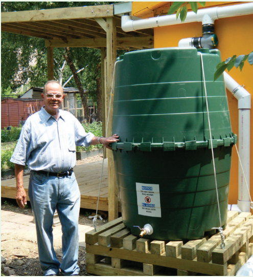
Rainwater harvesting tank at Garden of Happiness in the Bronx.
