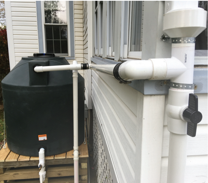
This RWH system on Staten Island required various PVC pipes and connecting pieces.
