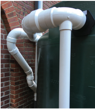
Elbows were used several times for this system.
